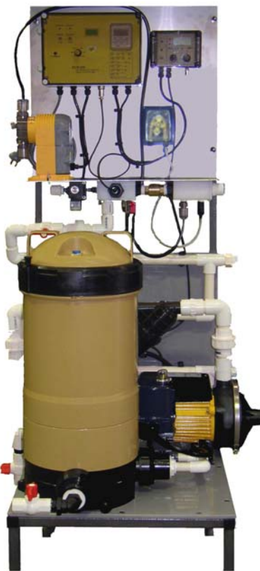
Bromine Canister System for Cooling Tower
